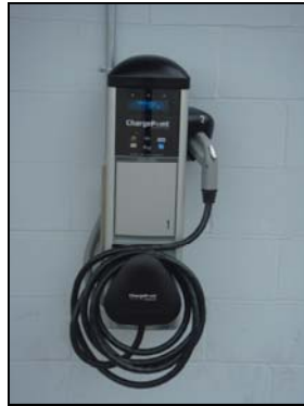
Level 1 (120V) and Level 2 (208V) Electric Vehicle Charging station.
